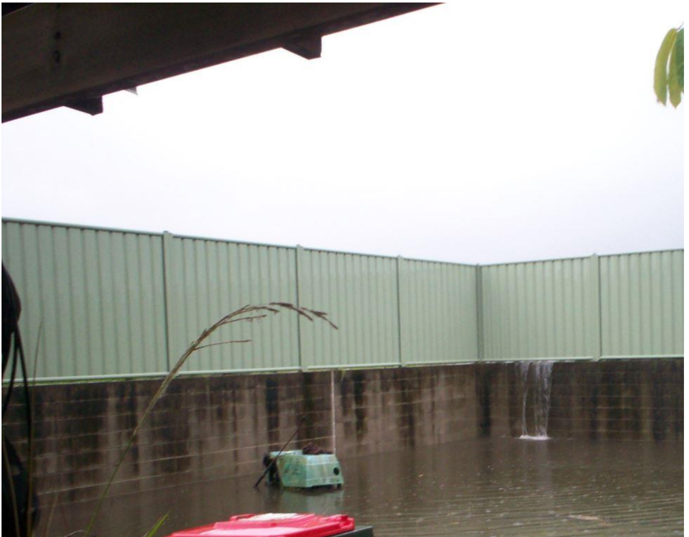
2. Backyard 127 Yamba Road – water pouring through retaining wall from Park Ave filled Subdivision site
