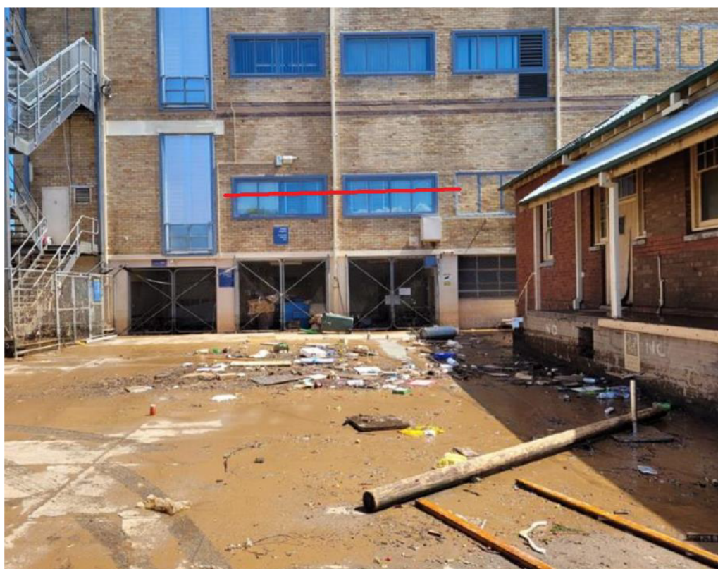
Figure 6: Lismore Exchange after flood waters had receded. The red line shows the high-water mark.
