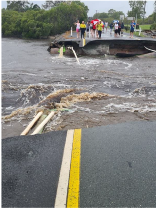
Figure 3: damaged fibre duct alongside a washed-out bridge, NSW/Qld border region
