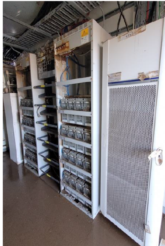
Figure 4: Flood-damaged mobile network equipment at Buckendoon (near Woodburn) in North-east NSW (See Case Study 2 below)
