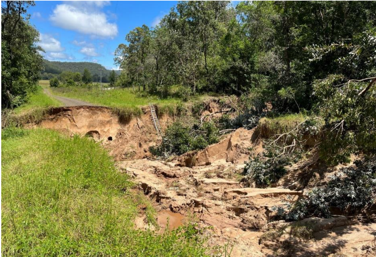
Council is facing more than $100m in major road repairs following the floods. This washaway on Upper Cherry Tree Rd, Mongogarie left residents isolated.
