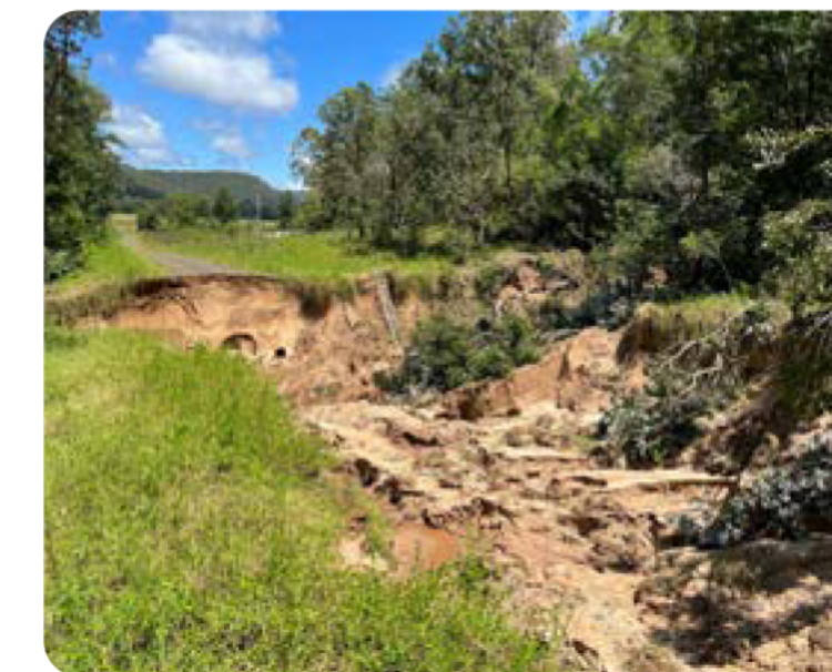
Severe damage to Upper Cherry Tree Rd, Mongogarie
