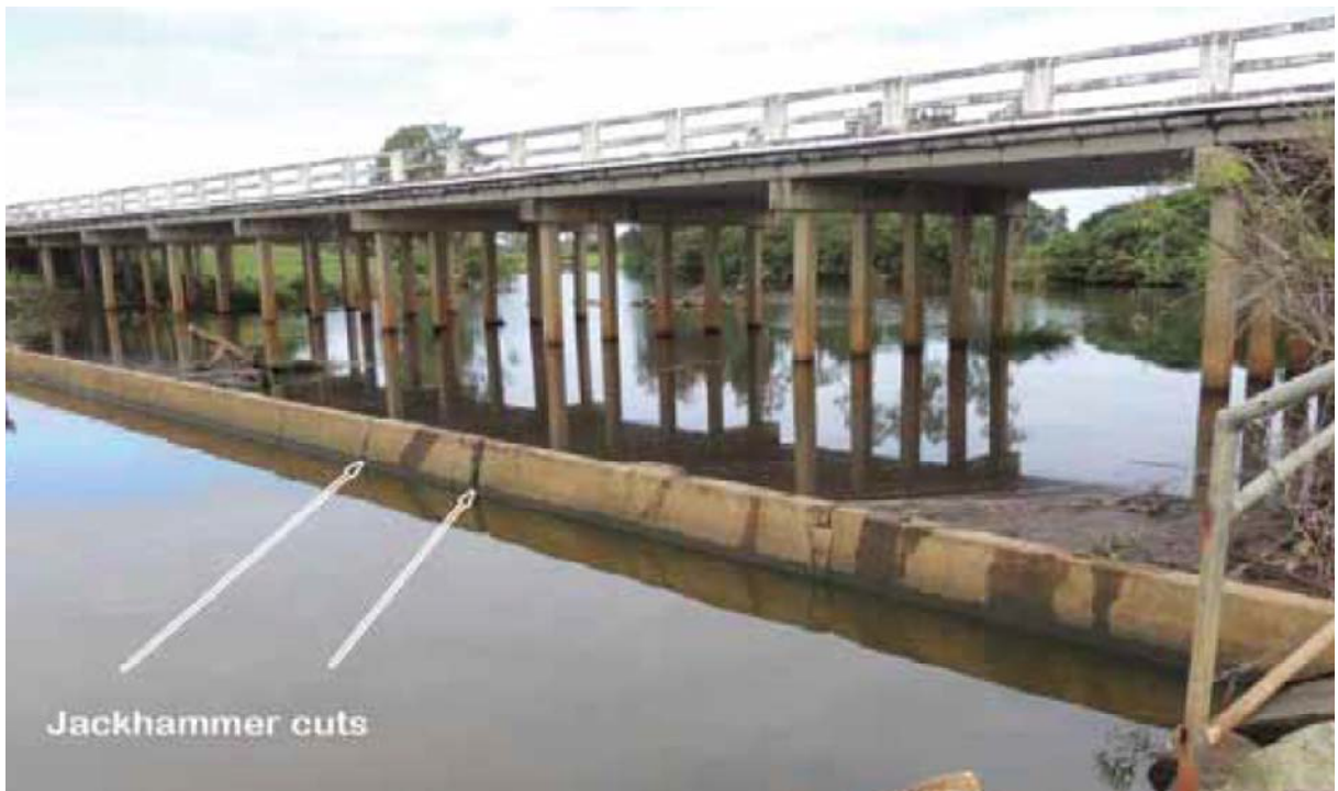
Fig 8 Damage to the fixed weir 2014
