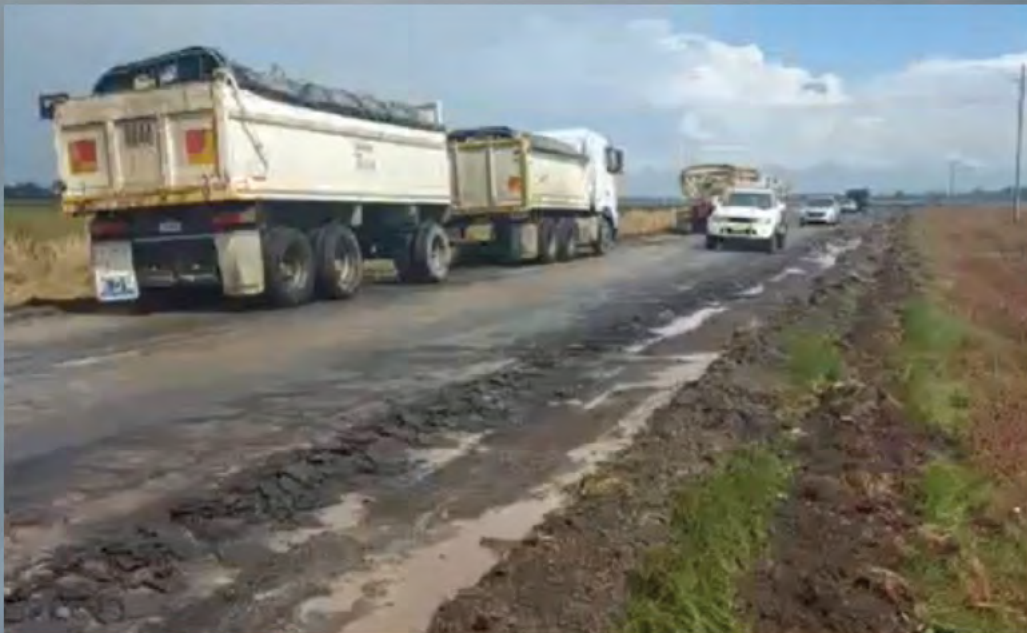
Coraki Road: Pavement damage caused by haulage of flood waste
