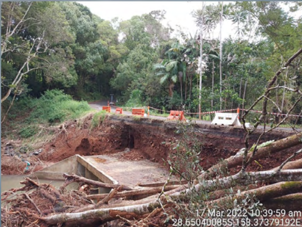
Dunoon Rd: Culvert washout
