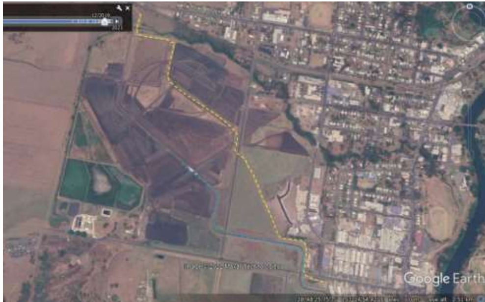
Figure 4. Earthworks (brown) nearing completion near the South Lismore sewerage plant (green), after moving 410,000m 3 of soil from the floodplain outside the levee to a development site inside the levee (levee shown as dashed yellow line), and intended to direct water via a zig-zag drain (dashed blue line) into the river below Lismore (bottom right of image).
