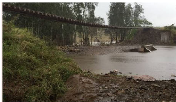
Damage to the rail line near Tocal. PHOTO: Cameron Archer
