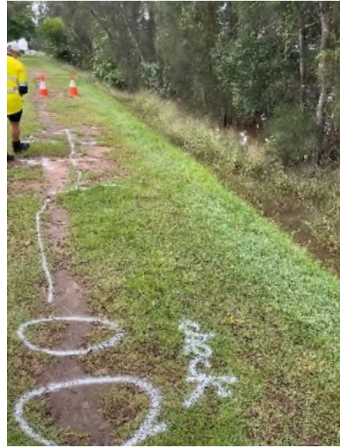
Crack observed on levee
