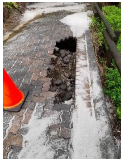
Scour on Marine Parade access to Main Beach
