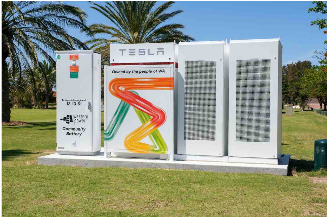
A community battery installed as part of a W.A. trial. Source: Western Power
