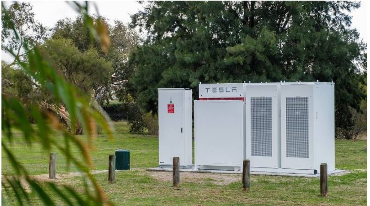
A community battery installed by Western Power in Western Australia. Image: Supplied
