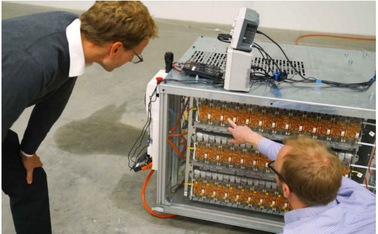
Relectrify's founders with a battery storage unit.
