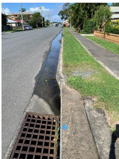
Image 4: Water run off to stormwater drain at [redacted] (May 2022)
