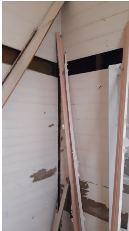
A board from every wall removed to allow for mould to be treated
