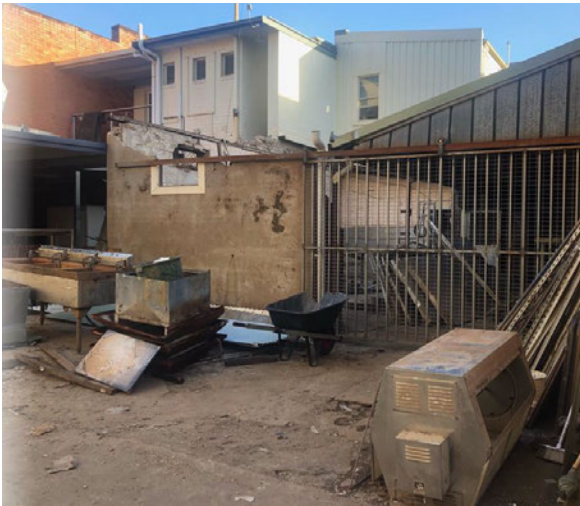
Post FEB 2022 – removal of Freezer from back alley way and demolition of roof and internal walls and disposal of unrepairable equipment
