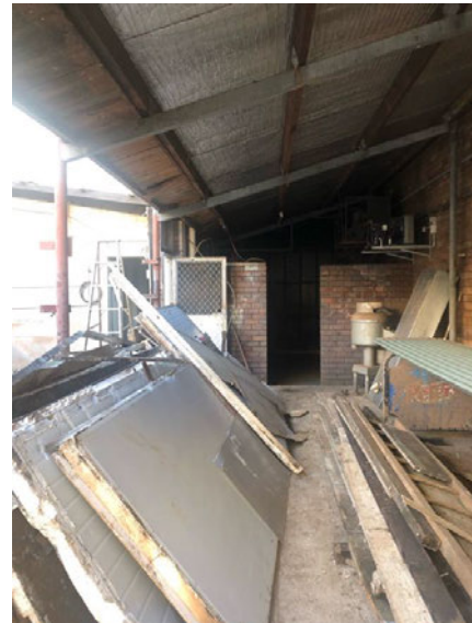
Post FEB 2022 – removal of Freezer from back alley way and demolition of roof and internal walls and disposal of unrepairable equipment
