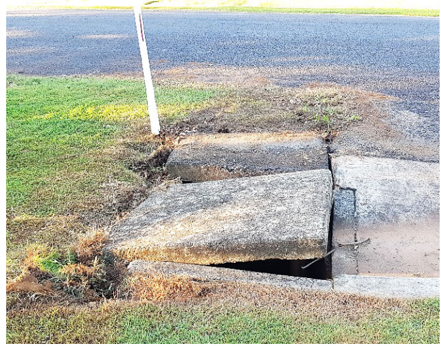
showing depth of wate at peak of flood..... and drain cover after flood
