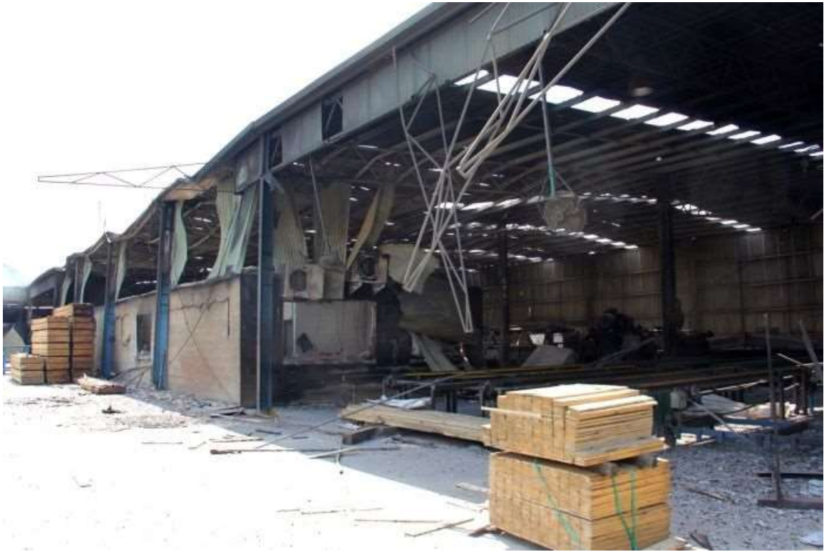
Figure 21 – Rappville sawmill destroyed by fire (source ABC)
