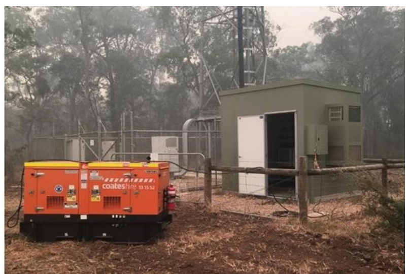
Figure 6: A generator at a mobile base station, Gelantipy VIC
