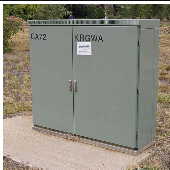
Figure 1: Example of a roadside cabinet
