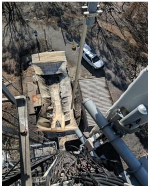
Figure 2: Fire-damaged mobile network facility, Mount Torrens SA
